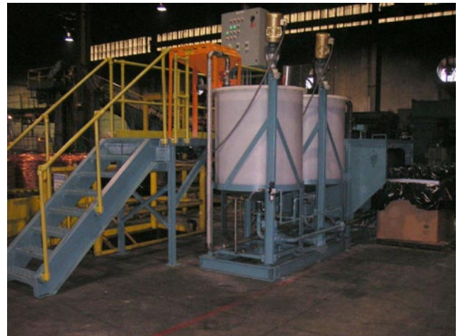
Figure 2 25 GPM (95 LPM) Treatment System
