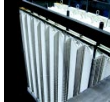
Installed Coalescing Plate Packs
