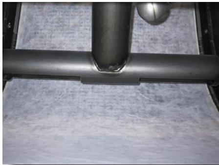
Dirty Inlet Distribution Header
