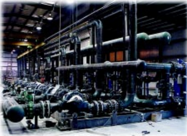
▲ Pump base for 1500 gpm tandem cold rolling mill.
