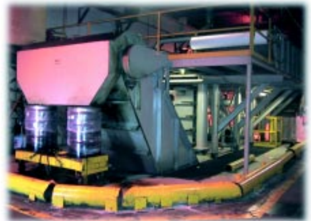
1000 GPM Continuous Cast ▲ Rod Rolling Filtration
